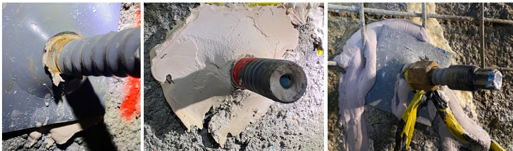
Figure 7 Polyethylene-coated dynamic MPA and Falcon bolts installed and grouted with polyester resin. The system provides full encapsulation with a high-strength grout, packing resin behind the plate and between the nut, which are common bolt corrosion locations
