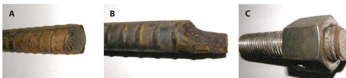
FIG 1 – (A) Rebar stress corrosion cracking; (B) localised pitting corrosion; (C) thread stress corrosion cracking.
