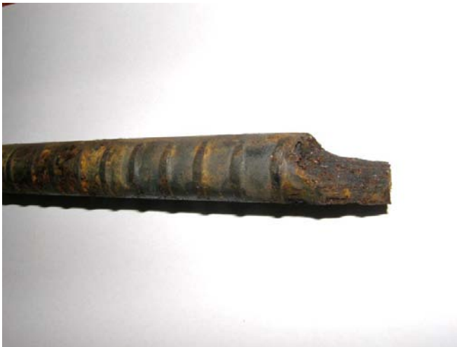
Figure 1b. Localised pitting corrosion.
