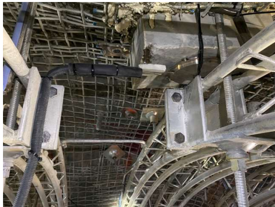
Figure 22 Example of radial pressure cell installed above the arch of the Lattice Girders
