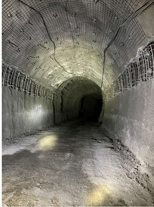
Figure 21 The Lattice Girders fully embedded into fibercrete, weld mesh is installed in the arch section
