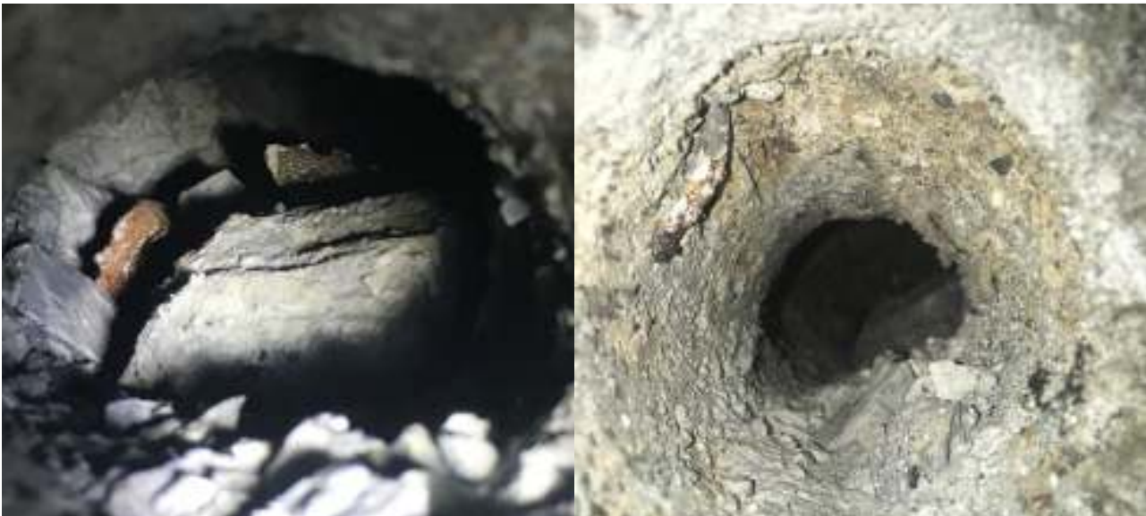
Figure 1 Typical hole conditions where the J-Lok P system is to be utilised, showing collapsed and 'blown out' drill holes. These are the type of ground conditions where traditional resin bolting is extremely difficult and time consuming
