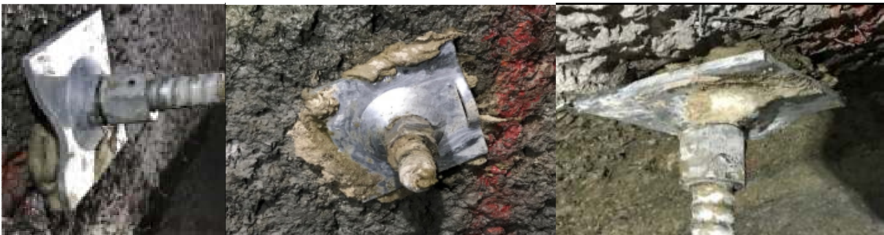
Figure 14 Installation of multiple R32 MPA bolt using the J-Lok P resin injection
